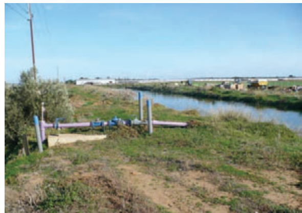
Figure 17.4. Recycled wastewater from the City of Adelaide, Australia, is pumped into an irrigation pond for a vegetable farm. Wastewater-conveying pipes are painted purple to distinguish them from freshwater conduits.
